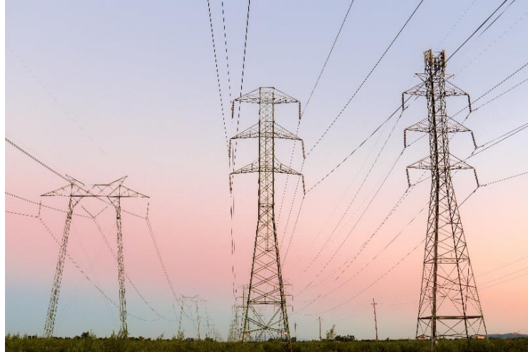
High voltage transmission lines move power from bulk generation to distribution power lines.
